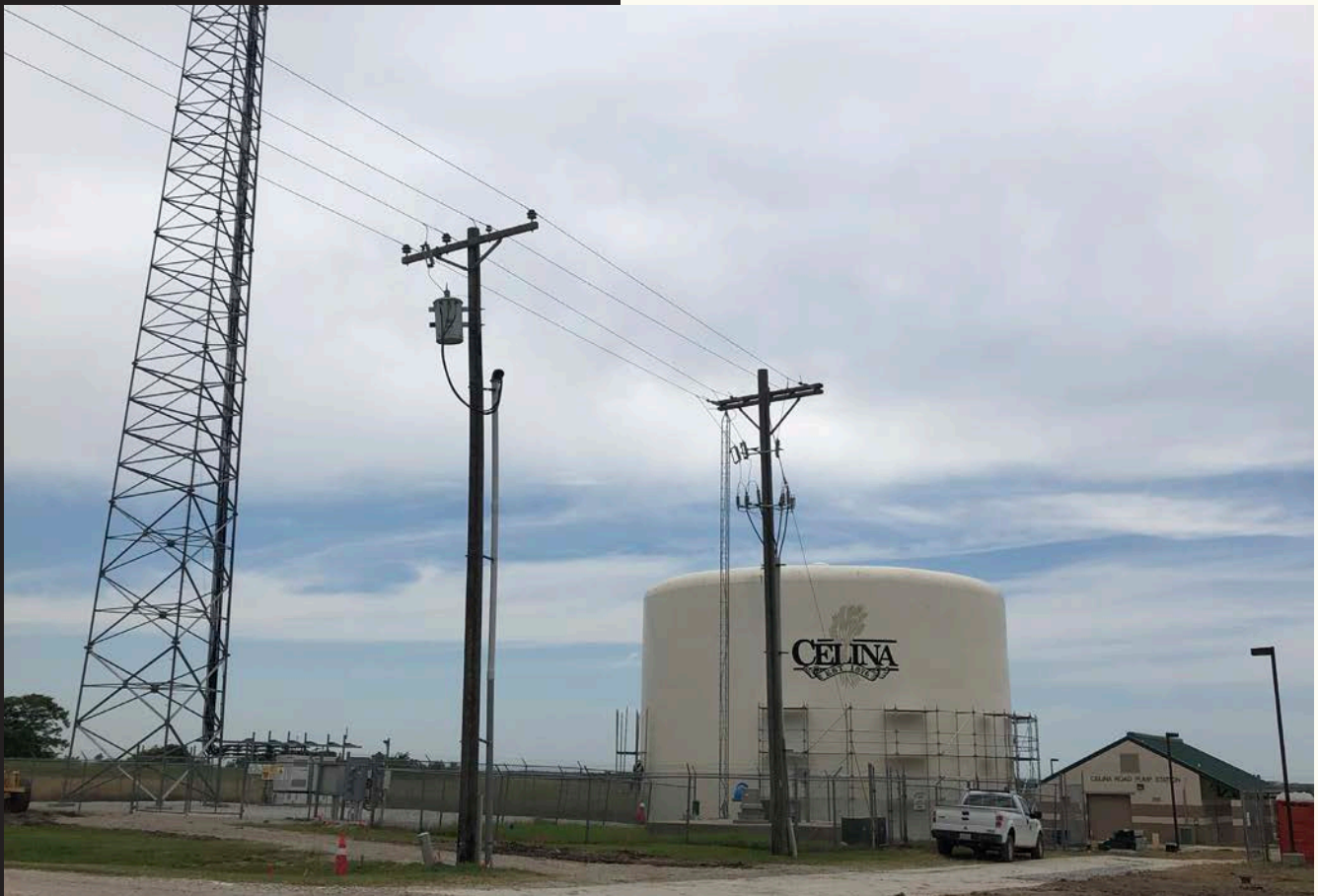
CELINA PUMP STATION
